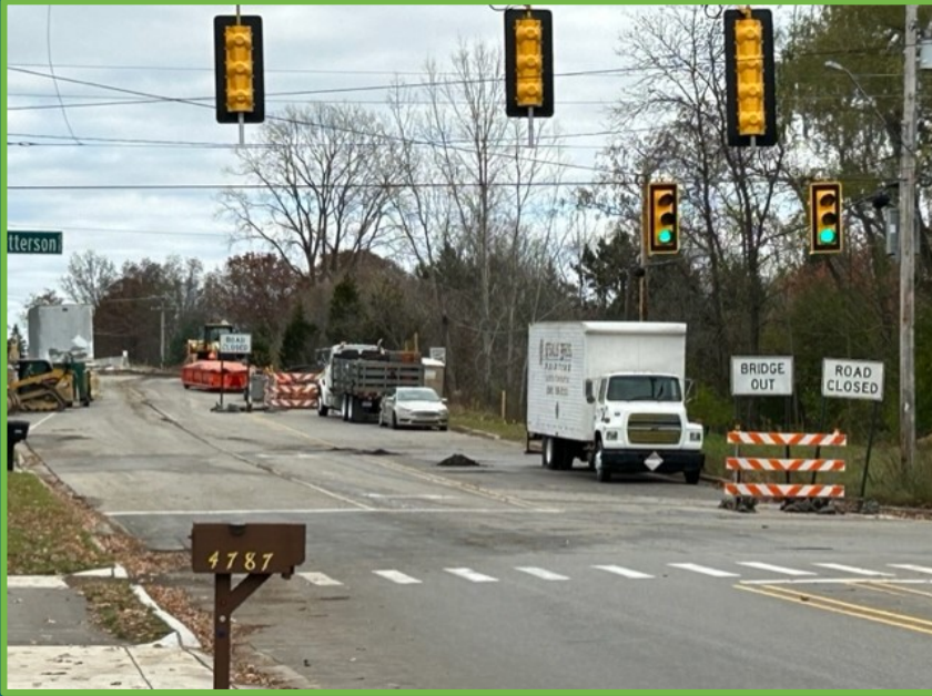
Burton St. Bridge Reconstruct over I-96 in Cascade Twp; Photo courtesy of GVMC Staff
