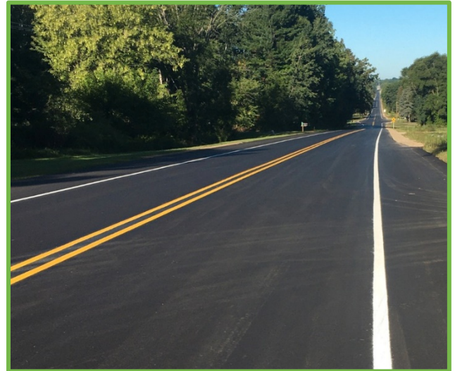
10 Mile Rd. Reconstruct West of Rockford; photo courtesy of Kent County Road Commission (KCRC)
