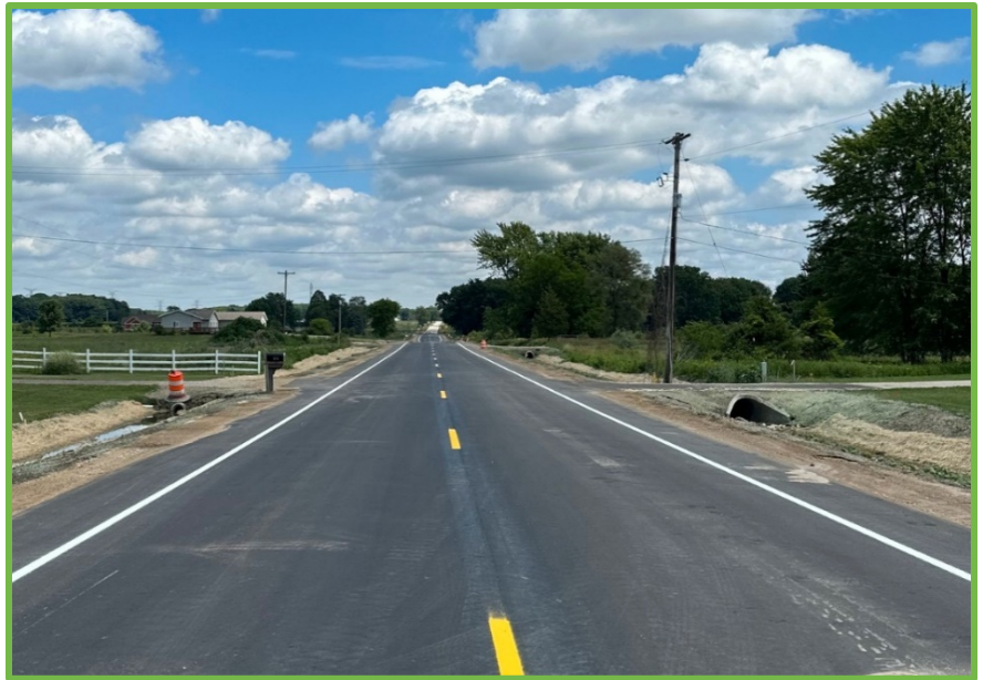
Construction on 84 th St. between Hanna Lake Ave & East Paris Ave in Gaines Twp; photo courtesy of KCRC
